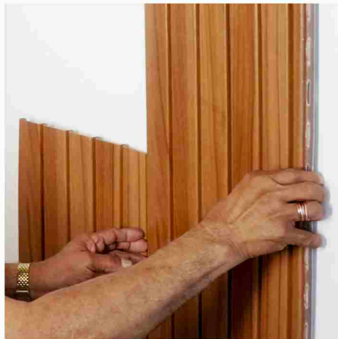
3. Take the second louver and interlock it with the first using 'Rapid-Clad' interlocking technology
